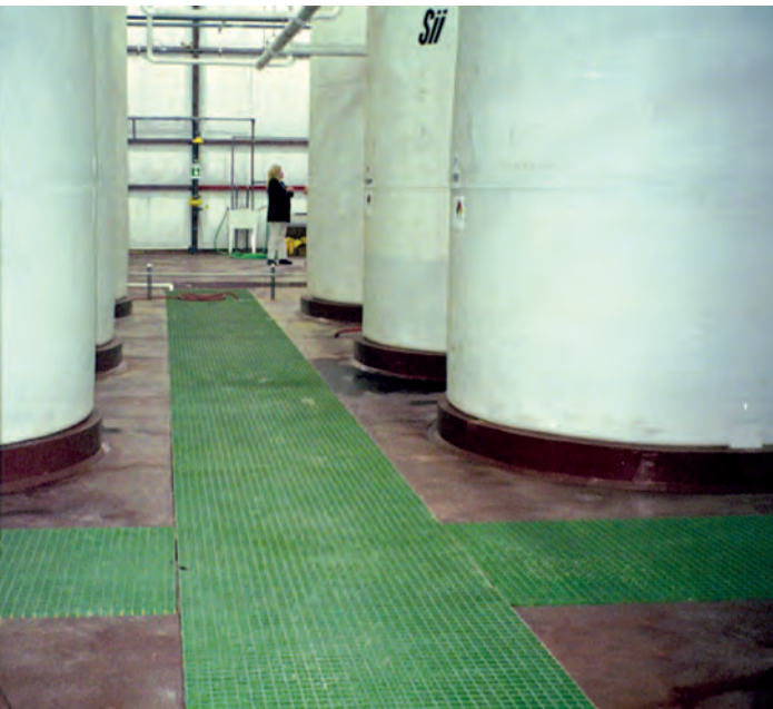
The Exide Battery Plant in Manchester, Iowa installed corrosion resistant DURAGRATE® around its tanks of sulfuric acid.
